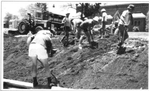
Voluntary workers contributed greatly to the successful completion of the Therry Centre
